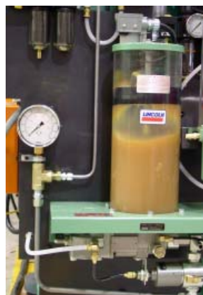
Pressure gauge at Pump
