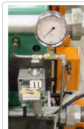
Pressure gauge and Pressure Switch at End of Line
